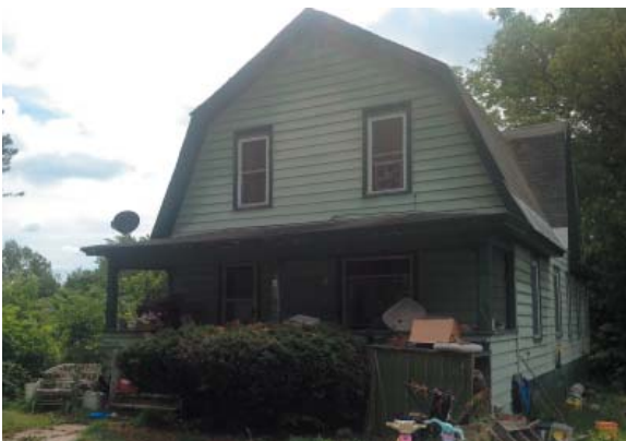
A single dominant roof form is clear, with secondary roofs covering the front porch and dormers.
