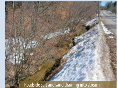
Roadside salt and sand draining into stream
